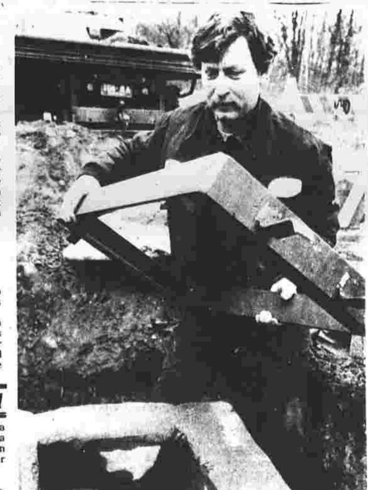
Water control Robert Oliver of the town Highway Division constructs a storm water catch basin on Birch Mountain Road on a recent afternoon. The catch basin is one of several being built in connection with work on the road.
